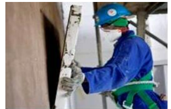
Wall Systems / EIFS
